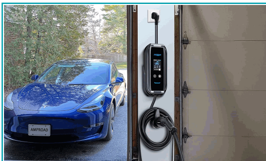
So Comfortable to Be a Garage EV Charger
