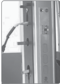
10 The length exceeds the door panel by about 2cm
